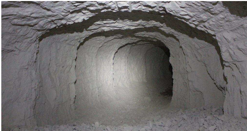
Figure 2. Tunnel that is currently being excavated to reach the underground site of the clock
